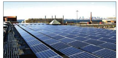
Broadway's design/build 456.12kW solar electric system project at MWRA's Winthrop treatment plant was completed in May 2011.
