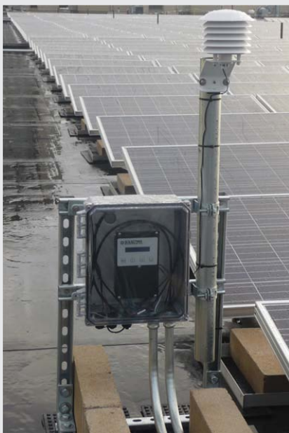
Solectria Renewables' weather station can withstand all weather conditions.
