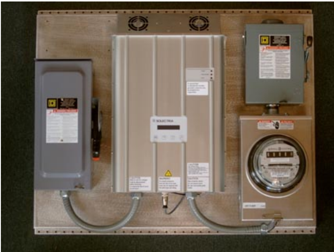
Fig. 7 A typical PVI 1800 or PVI 2500 installation with AC and DC disconnects. (AC disconnect is on the right, DC disconnect on the left. PVI 2500 shown.)
