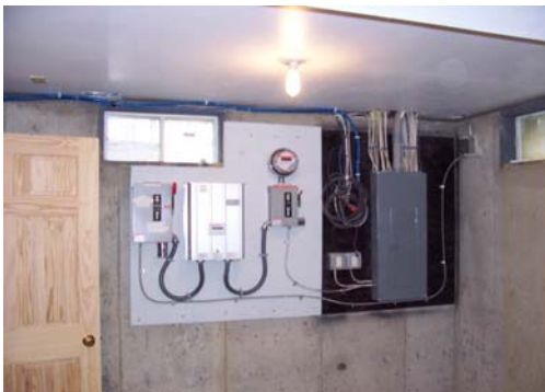
Painted plywood board in basement (BPVS)
