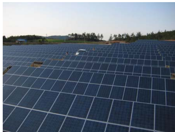
Array at 1.2MW HaeNam Site (HHI Modules)
