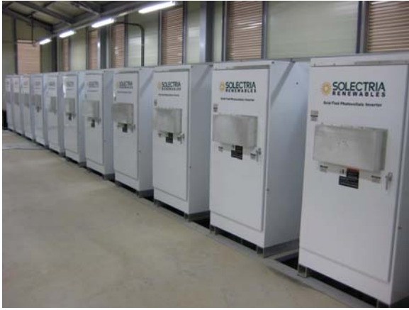
Jeongeup PV System 1.6 MW
